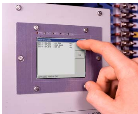
Touchscreen LCD allows fault teams to access recent data on site
